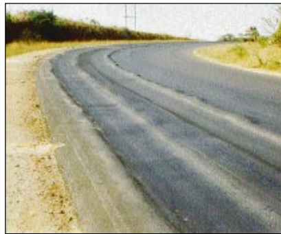
Early surfacing failure
