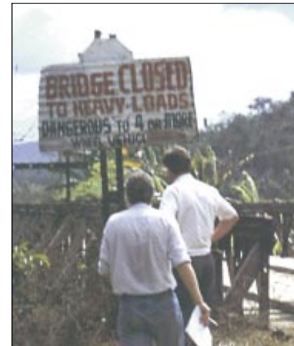
Philippine transport is frequently overloaded, and some older steel bridges are showing signs of distortion and dangerous corrosion
