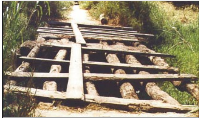
Local authority built bridge, suffering from lack of maintenance
