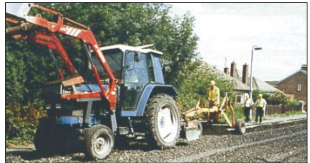
Tractor equipment used in the rehabilitation of bituminous surfaced pavements in the UK
