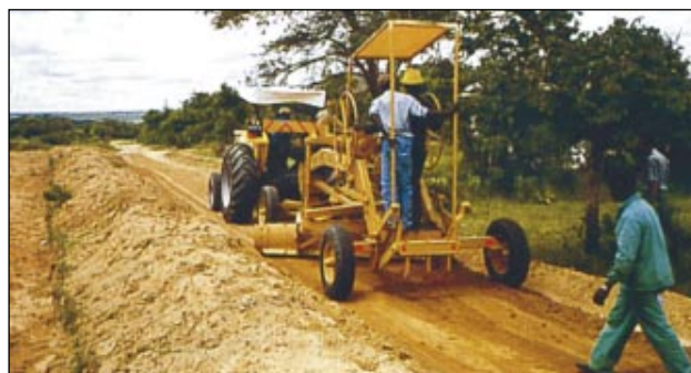
Light towed grader extensively used for routine maintenance of unpaved roads in southern Africa
