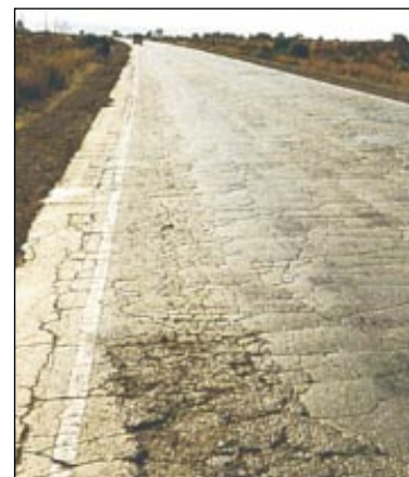
A severely cracked road in Africa - can it be recycled?
